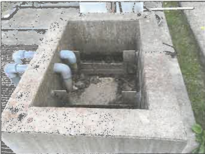
Equalization Basin (Splitter box)
