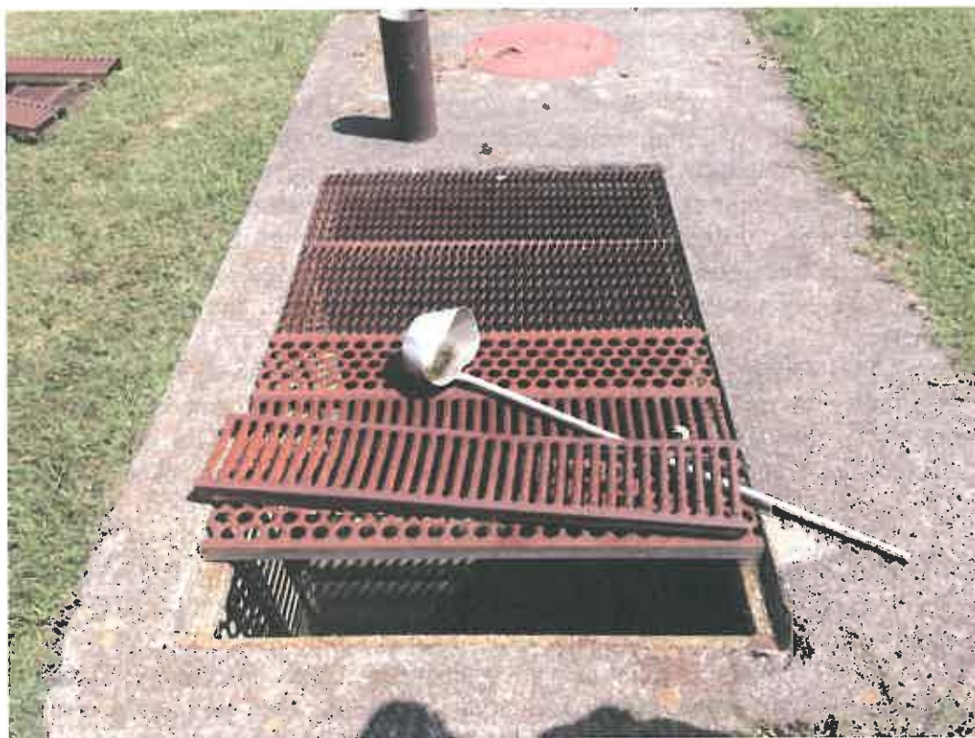
Wastewater Treatment Facilities at Canaan Valley Resort State Park Photo by Dunn Engineers, Inc. 2016 for Report to DNR See APPENDIX C
