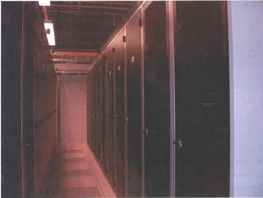
Figure 2 – Dallas Level 3 NICE inContact Locked Cabinets
