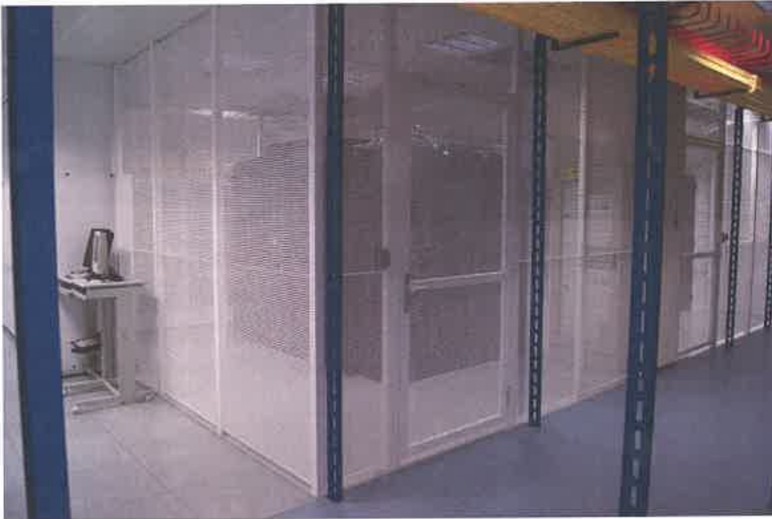
Figure 3 - Germany Equinix NICE inContact Locked Cage
