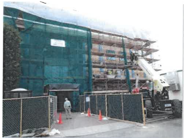
Overhead protection for building occupants at the entrance to the Public Service Commission Headquarters Building during construction
