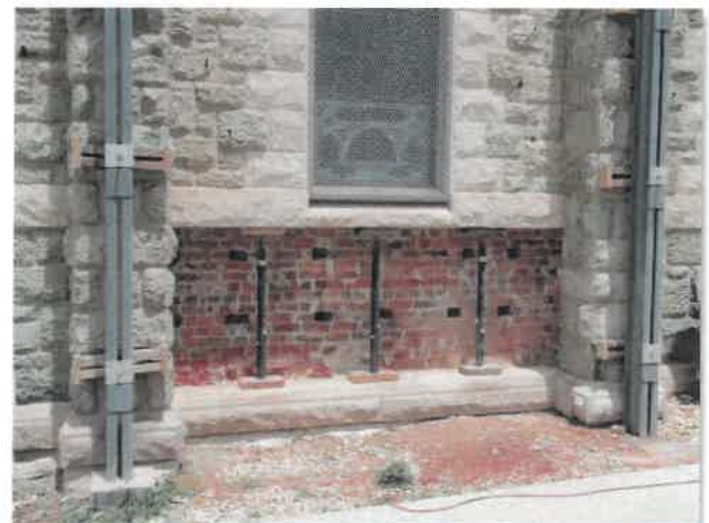
Exterior support buttresses and existing wall section removal at St. Francis restoration
