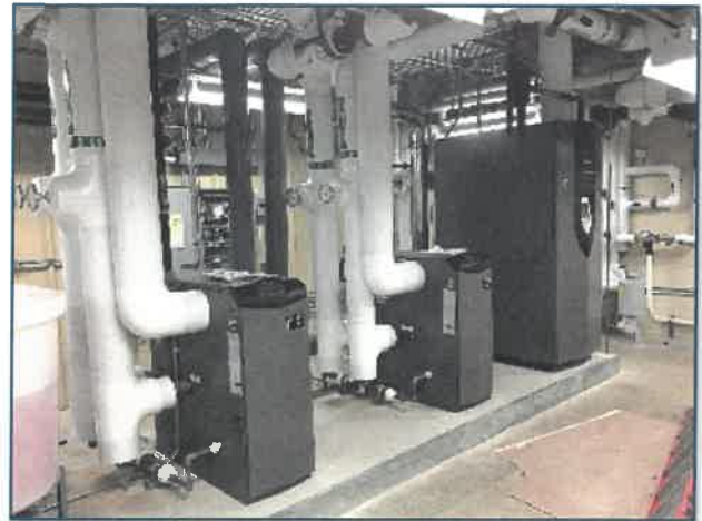
High Efficiency Boilers
