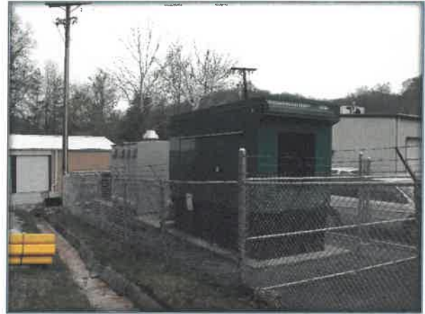
Diesel Electric Generator
