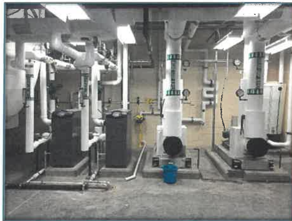
High Efficiency Hot Water Boilers and Pumps
