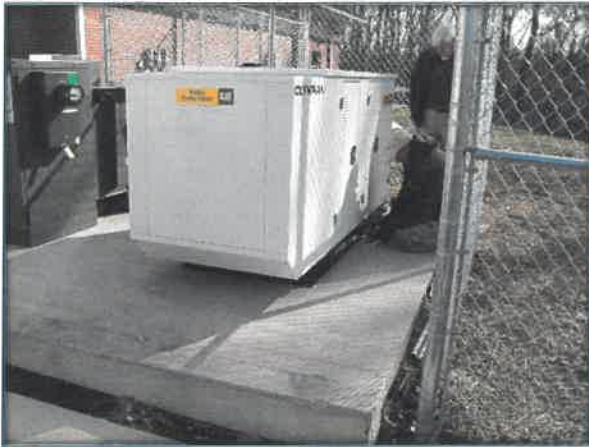
Natural Gas Electric Generator
