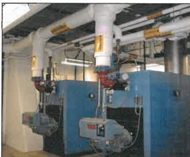
New Boiler Plant
