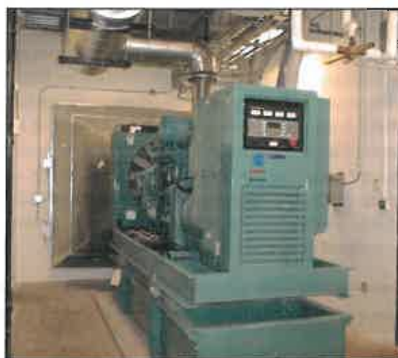
New Emergency Generator
