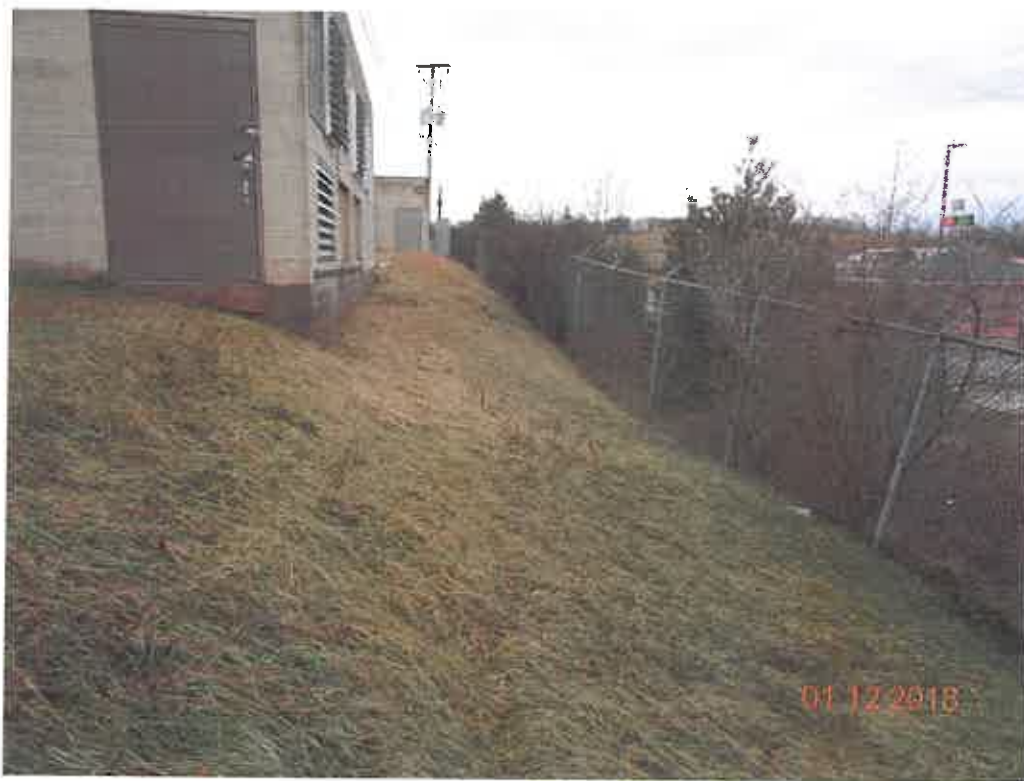
Overall View of Landslide Area
