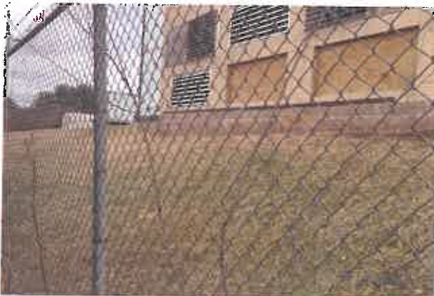
WVDA Warehouse Slope Slippage
