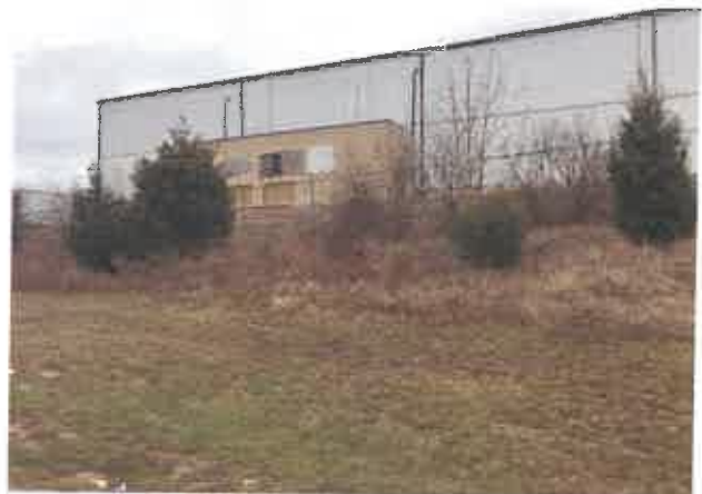
WVDA Warehouse Slope Slippage
