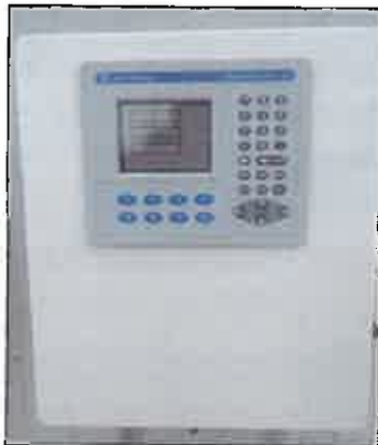
Remote Truck Fill HMI
