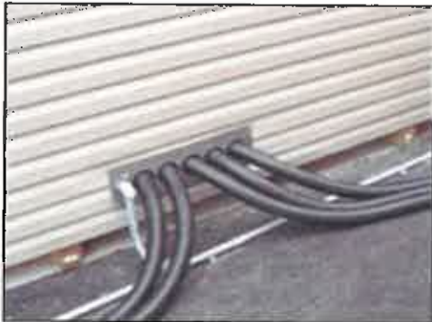
Ex 1: Wall plate used for thru-wall hose run
