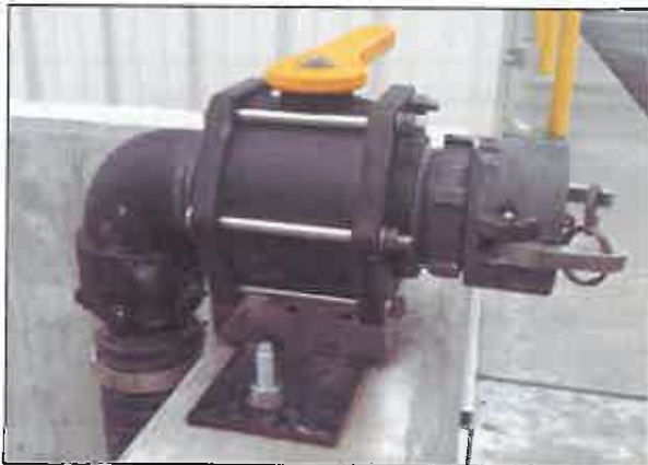
Truck Filling Station setup(hose connecting to tanker truck not shown)
