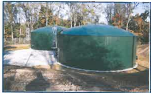
New Water Storage Tanks near Ceredo, WV
