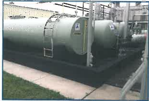
NiSource Aboveground Storage Tanks
