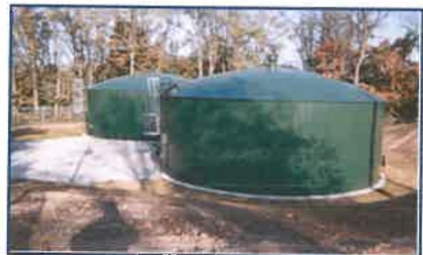
New Water Storage Tanks near Ceredo, WV
