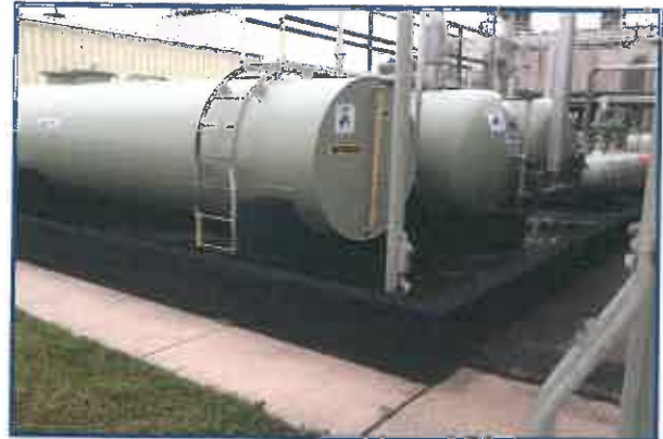
NiSource Aboveground Storage Tanks
