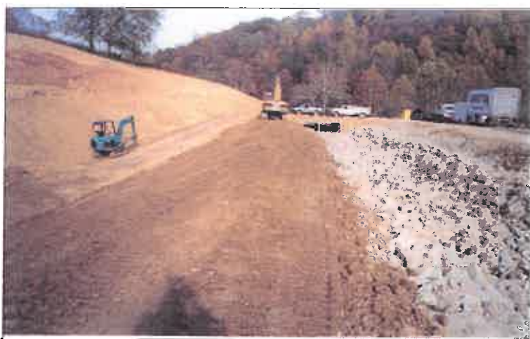
The emergency spillway from the sediment pond drains to a riprap-lined channel and through a box culvert.
