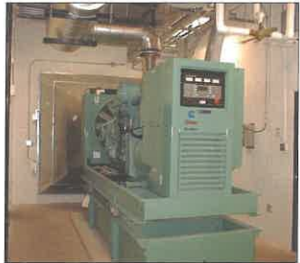
New Emergency Generator
