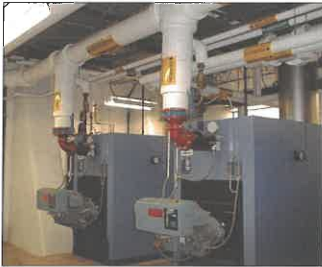
New Boiler Plant
