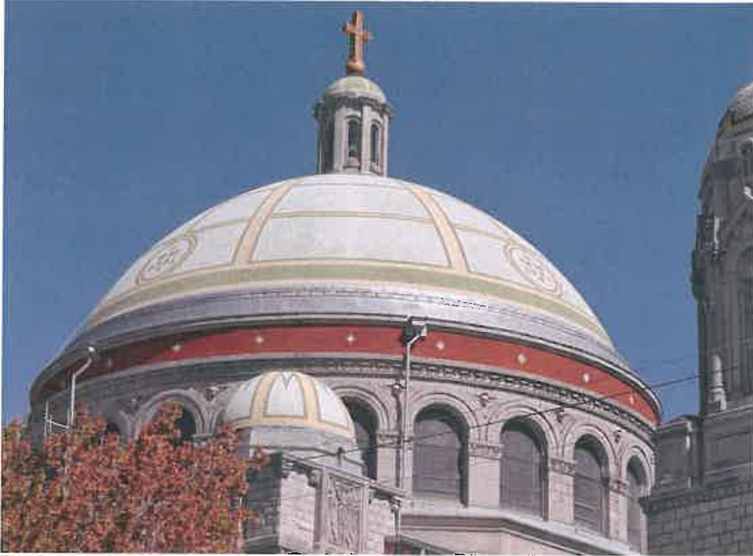
The Restored Dome, new gutters and metal roofs improve the Church's stormwater management.
