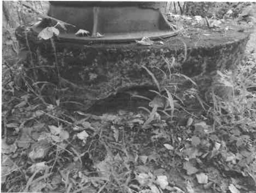
Manhole Identified for Replacement
