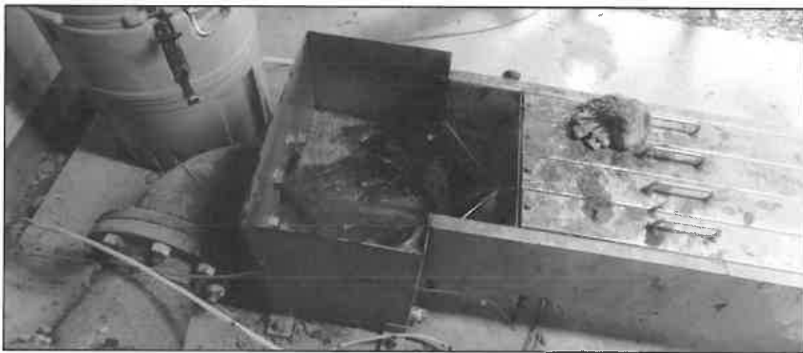
Existing UV Unit
