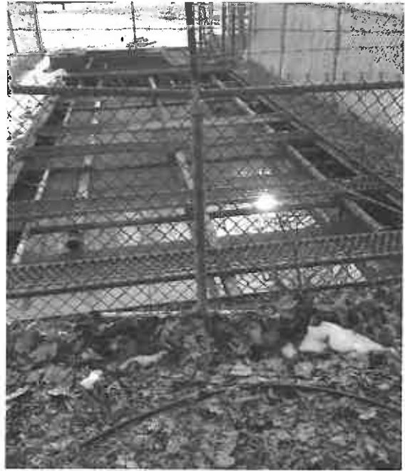
Failing Package Treatment Plant
