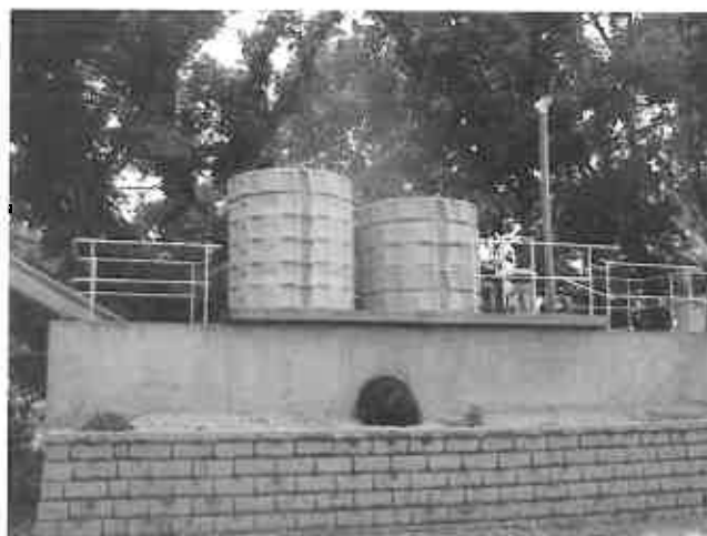
“Headworks” Facility with Scrubber Unit
