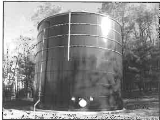
402,000-Gallon Water Storage Tank
