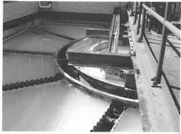
Upflow Clarifier Prior to Replacement
