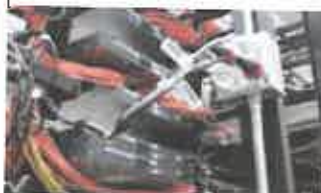
Cable run in server room.
