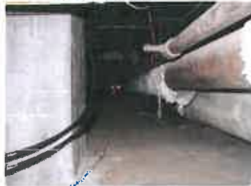
Friable Asbestos Pipe Insulation
