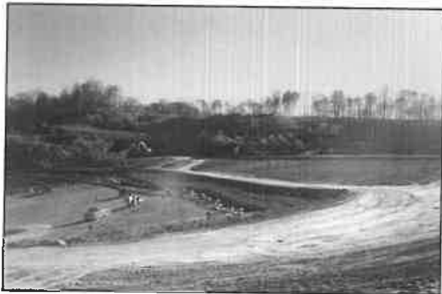
Construction of the cap system was completed in phases. A buttress was constructed over the face of the landfill to flatten slopes to 4 horizontal to 1 vertical to improve stability of the cap.
