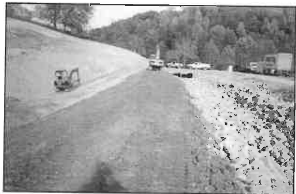
The emergency spillway from the sediment pond drains to a riprap-lined channel and through a box culvert.
