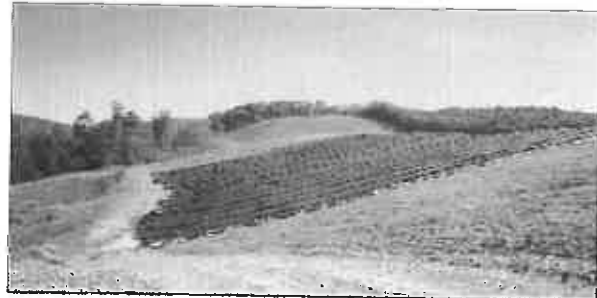
Cell 1-B slope covered with geosynthetic cap prior to placing the final soil cover layer.
