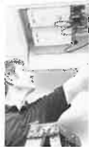
Access point enclosure in hospital hallway.
