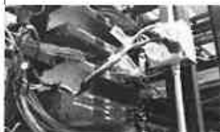
Cable run in server room.
