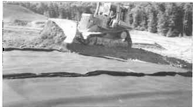
A bulldozer was used to place the 2-foot thick final soil cover layer working from the bottom of the slope to the top.
