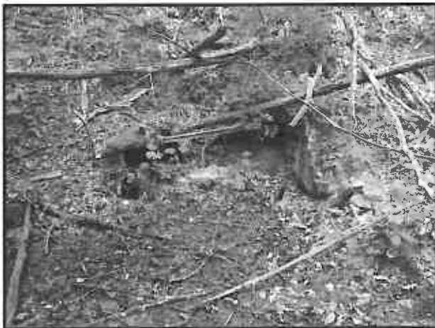
Collapsed Portal Structure
