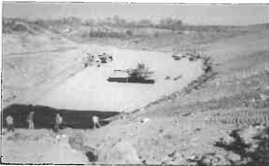
Construction of the 60-mil HDPE geomembrane over the prepared soil subgrade and excavation of perimeter anchor trenches.
