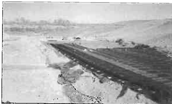
HDPE drainage net was installed as the leak detection layer above the 60-mil HDPE geomembrane.
