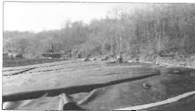
HDPE geomembrane was covered with HDPE drainage net to serve as the leak detection and leachate collection zones.
