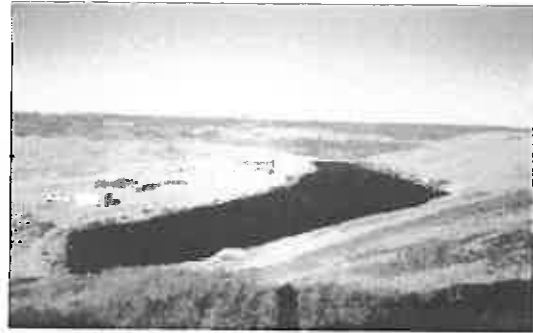
Completed geosynthetic liner system of Cell F-3b ready to receive the protective soil cover.
