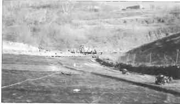
Placement and seaming of 80 and 60 mil HDPE geomembrane was included in the new cell.
