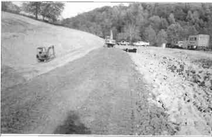
The emergency spillway from the sediment pond drains to a riprap-lined channel and through a box culvert.
