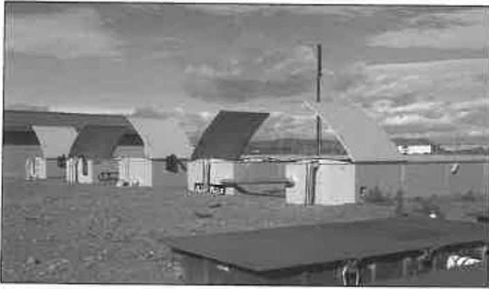
The Yakama Nations Housing Authority in Washington state added five AdvanTex ® AX-Max units (background) to its ten AdvanTex AX-100 units, increasing the capacity of its wastewater system by 50%. Photo courtesy of Fextex Systems, Inc.
