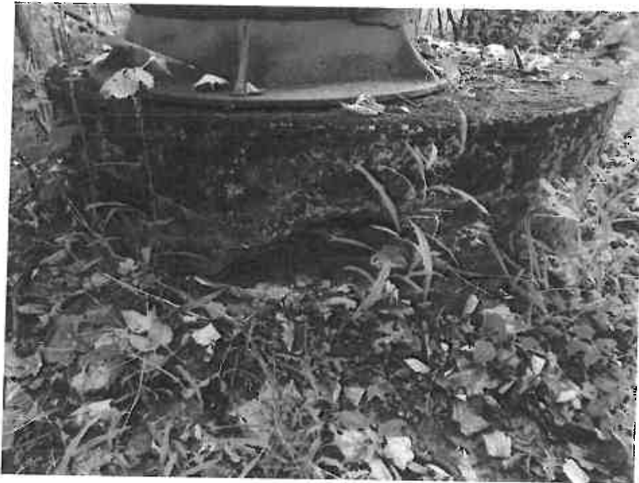
Manhole Identified for Replacement
