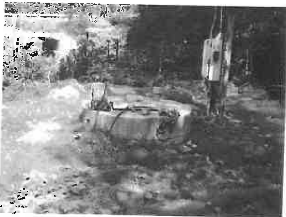
Before: Upper Drive Lift Station
