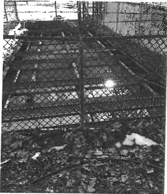
Failing Package Treatment Plant
