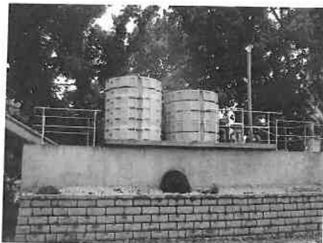
"Headworks" Facility with Scrubber Unit
