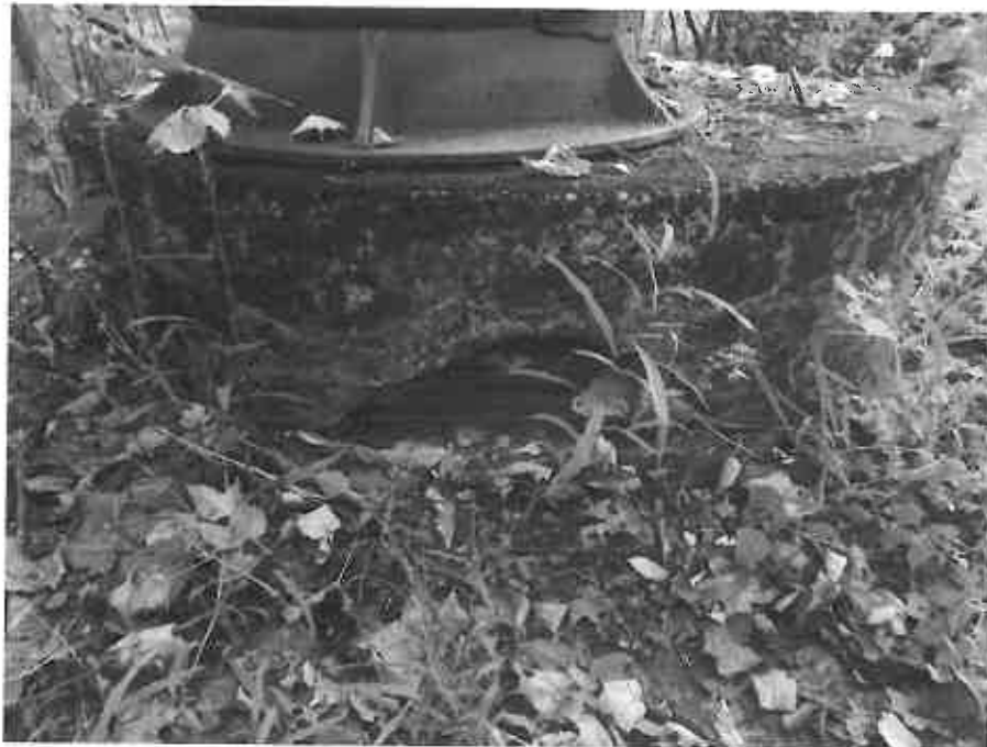
Manhole Identified for Replacement
