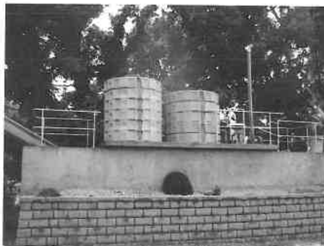
“Headworks” Facility with Scrubber Unit
