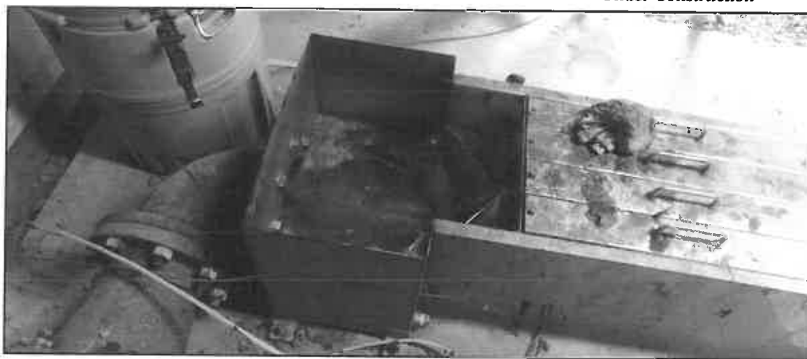
Existing UV Unit
