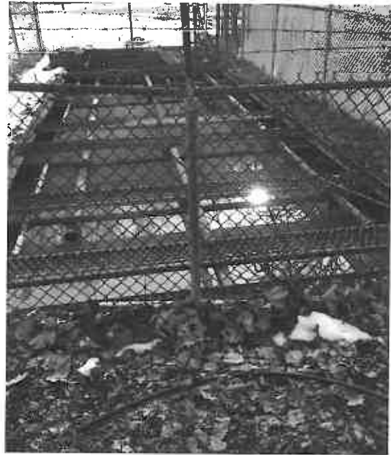
Failing Package Treatment Plant
