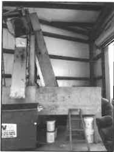
Mechanical Bar Screen to be Replaced
