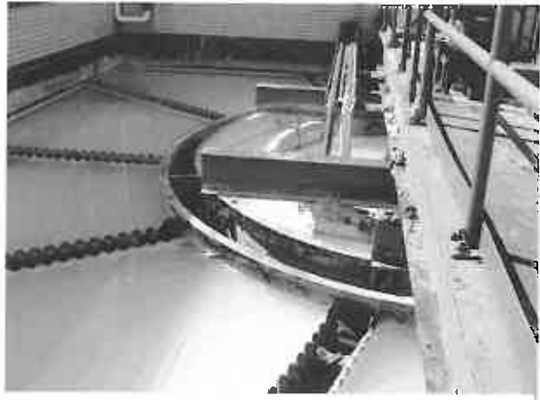
Upflow Clarifier Prior to Replacement
