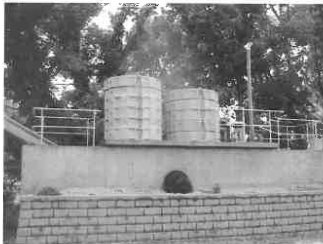
“Headworks” Facility with Scrubber Unit
