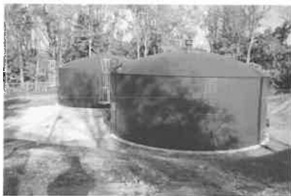
Two new water storage tanks.
