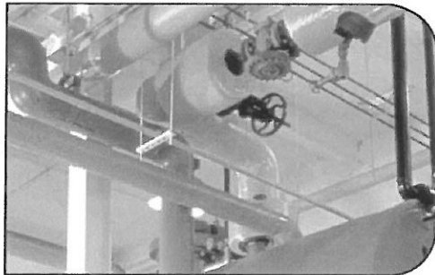
(top) Split Rock Pools—Snowshoe, WV Piping & Pump Room
