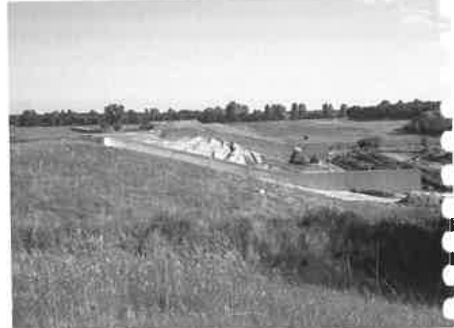
Renwick Dam. A key feature of this rehabilitation project is a stepped, RCC spillway over the embankment.
