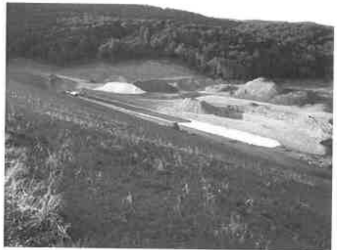
Figure 27: New Creek Site 14 Fine and Coarse Drain Fill Placement. Our experienced fill/excavation inspectors were on site during placement of fill/drainfill at New Creek Site 14.
