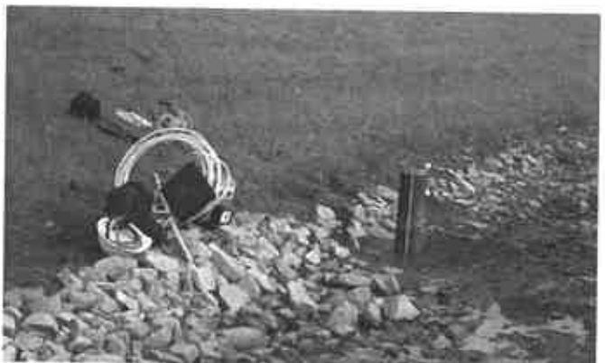
Hibernia Dam. Gannett Fleming performed investigations, evaluations, monitoring, analysis, and interpretation of elevated piezometer readings to assist in the determination of cause and effects for the higher than normal piezometric readings.
