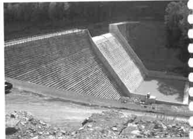
Elkwater Fork Water Supply Dam. NRCS chose Gannett Fleming for this project because of our experience; our capability to design the project within a constrained construction schedule and funding limitations; and our ability to provide comprehensive geotechnical, environmental, and drilling services throughout investigation, design, and construction phases.
