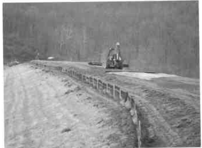
Figure 26: New Creek Site 14 Pollution Control Measures. We inspected erosion control measures for the access road along the crest of dam for the multi-year construction project at New Creek Site 14.
