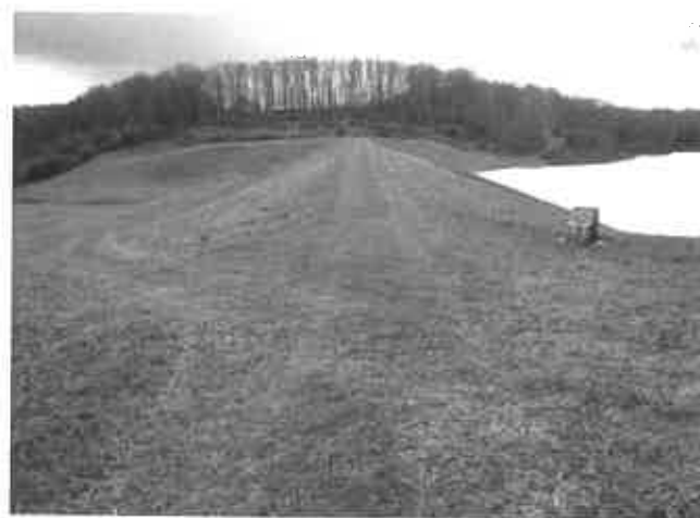
Upper Deckers Creek Site 1. To comply with Class C high Hazard design criteria, Gannett Fleming recommended excavating an earth/rock cut auxiliary spillway at the left dam abutment appeared to be the most economical alternative for both maintaining the existing pool and raising the pool to provide additional water supply storage
