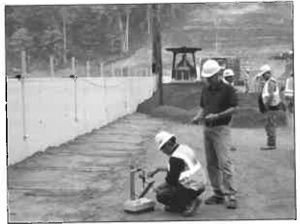
Figure 23: Elkwater Fork Dam. Gannett Fleming oversaw quality control testing of RCC at NRCS WV's Elkwater Fork Dam.
