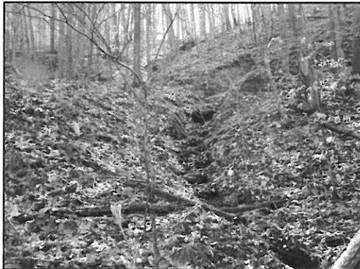
Eroded drainage path from bench
