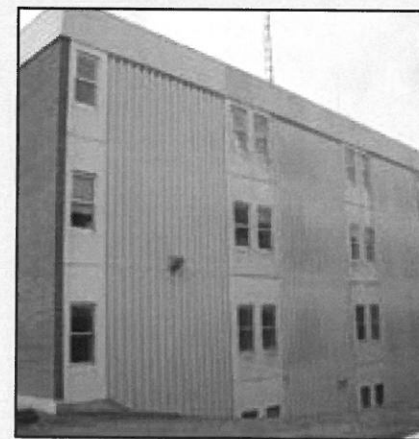
Old Mount View High School windows prior to replacement.
