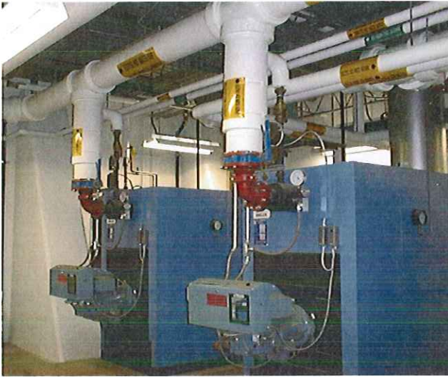
New Boiler Plant
