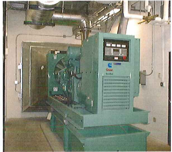
New Emergency Generator
