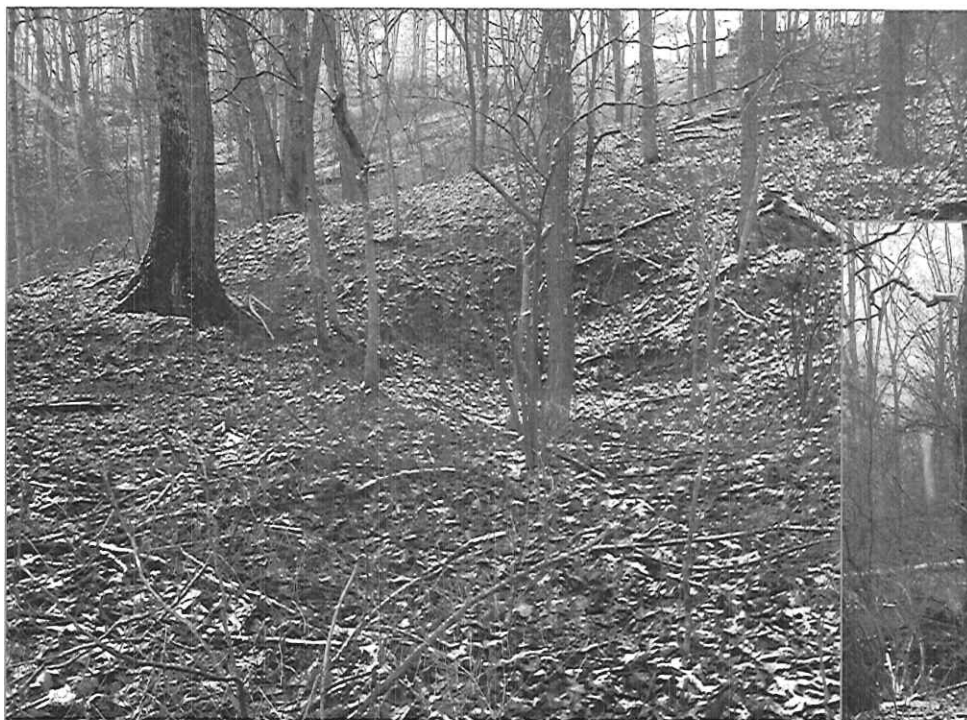
Photo "D" – Larry Frederick Slump Area
