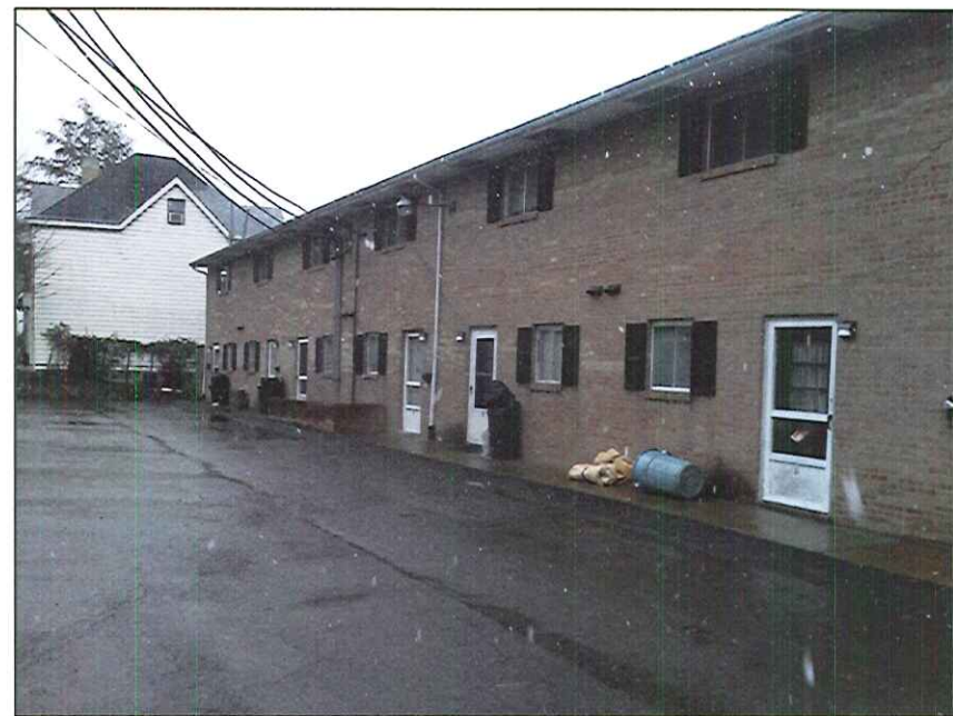
Photo E – Effects of Subsidence "Cracks in Structure"
