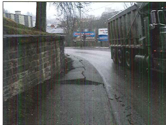
Photo H - Impacted Road
