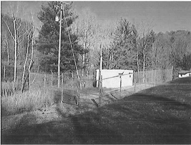
50 GPM Wilsontown Booster Station
