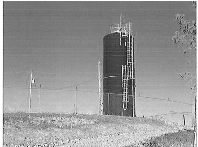
43,000 Gallon Salem Ridge Water Storage Tank
