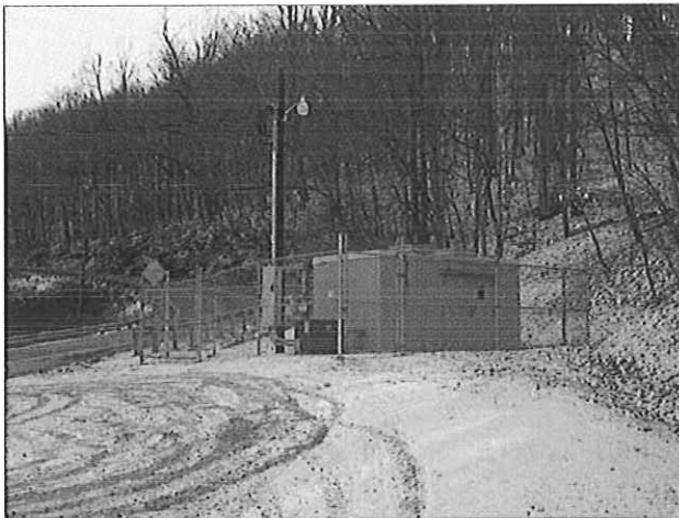
250 GPM Water Booster Station on Route 20
