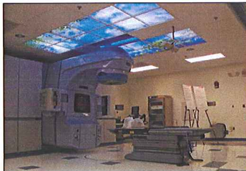
Mount Nittany Medical Center. A new linear vault was added to replace the original linear accelerator vault.
