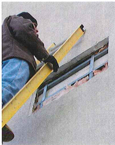
At West Park Court, samples of the existing EIFS finish were removed to expose supporting sheathing and subsurface conditions—a typical first step in PWWG's forensic assessments.
