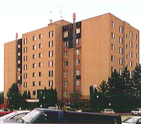
St. Theresa Plaza (Pittsburgh), where EIFS curtain walls on the 15 year old apartment building were cracked and damaged beyond repair. The new walls are constructed of durable pre-finished aluminum installed entirely from the outside.
