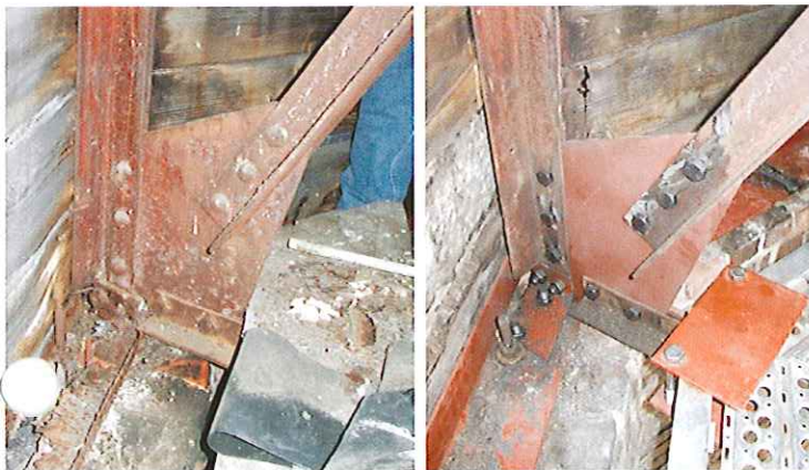
Left: Failed steel channel and riveted connection at truss. Right: Repaired connection at truss.
