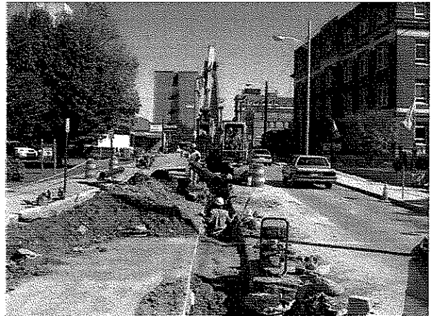
Completed in 2003 Main Street Waterline Replacement Project New 12" Ductile Iron Pipe Installation
