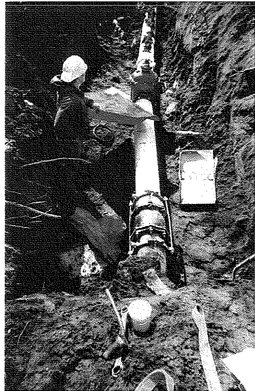
Connection of 10" HDPE River Crossing Pipe (Directionally Drilled) to 10" C-900 Pipe at Tygart Valley River
