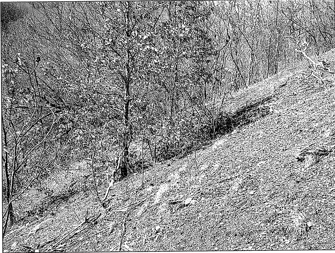
McCOMAS (POCA LAND) REFUSE PILE – MERCER COUNTY LOOKING DOWN HOLLOW FROM ROAD AT TOP OF REFUSE PILE
