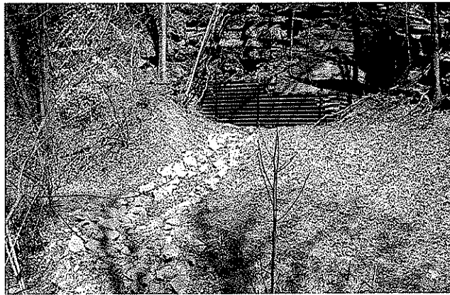
Bat Gate with rip rap channel
