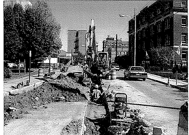
Completed in 2003 Main Street Waterline Replacement Project New 12" Ductile Iron Pipe Installation
