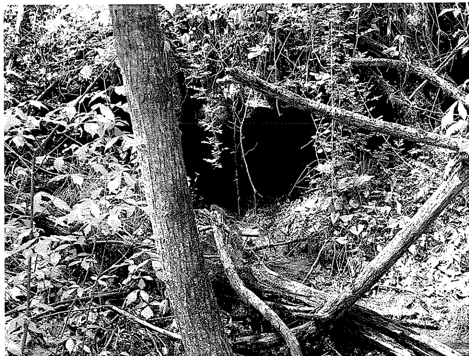
Picture 2 shows an open and draining portal at Site 1.
