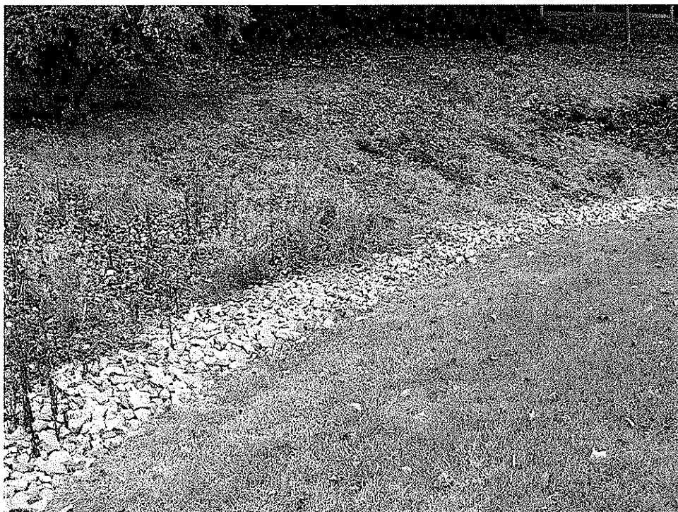
French drains installed behind residences in the area of the project site
