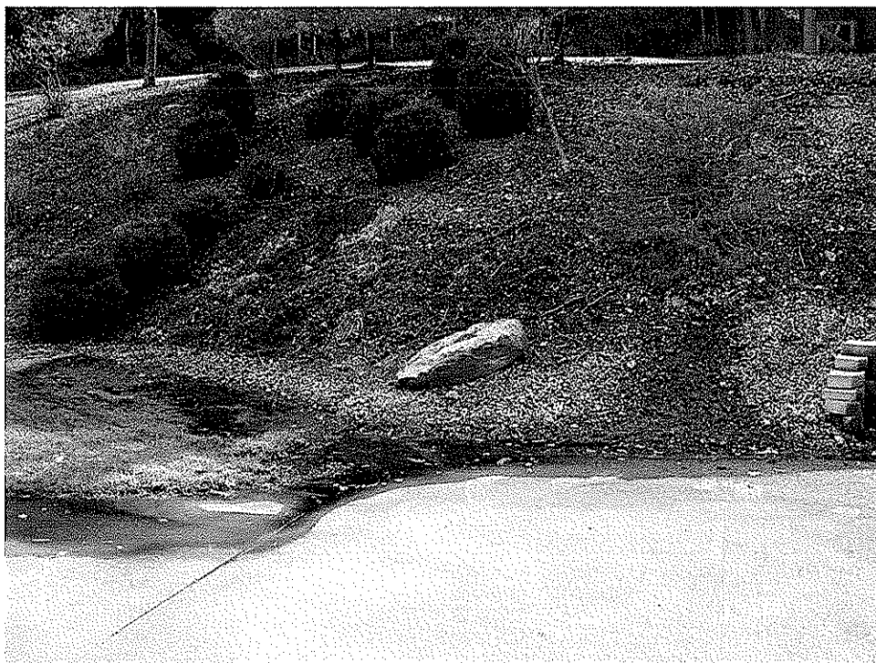
Seep at the driveway of 3961 East Lake Drive
