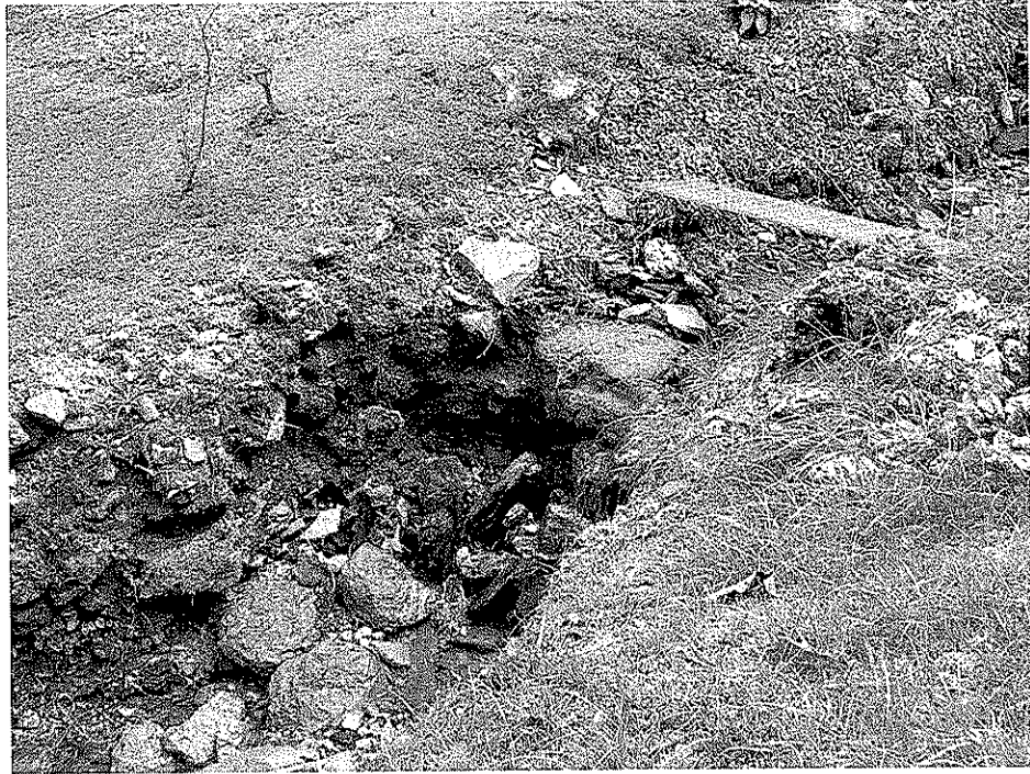
Picture 2 is debris that has eroded from the refuse pile and is clogging the stream.
