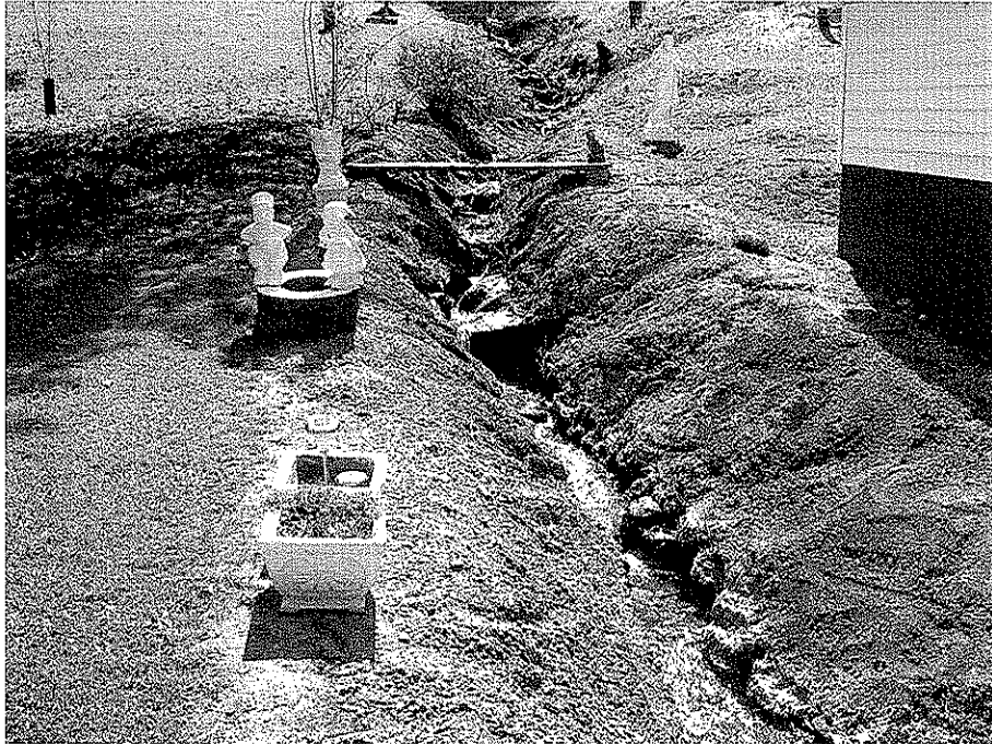
Picture 4 shows homeowner stream repairs. Note undermining of the concrete lining.
