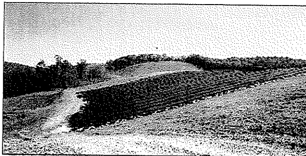
Cell 1-B slope covered with geosynthetic cap prior to placing the final soil cover layer.
