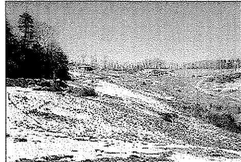
Portions of the landfill were steeply sloped which presented a challenge in designing the geosynthetic cap system.
