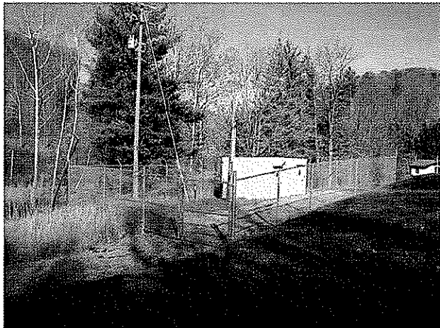
50 GPM Wilsontown Booster Station
