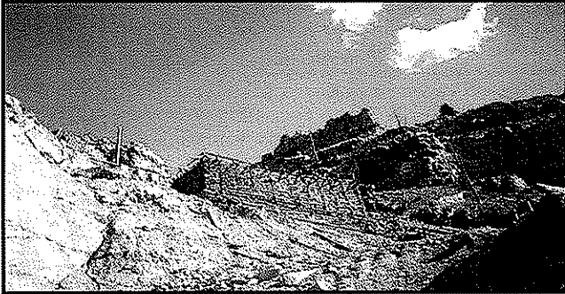
Remedial actions at the Eagle Mine site included plugging of adits to reduce acid mine drainage.
