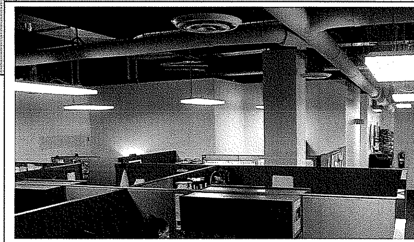
Photo Courtesy of ALPHA Associates
