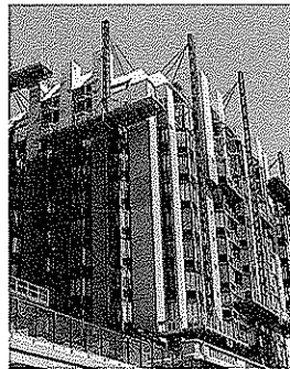
TWIN RESIDENTIAL TOWERS WJE INVESTIGATED LEAKAGE OCCURRING THROUGH WINDOWS AND EIFS CLADDING, AND RECOMMENDED RECLADDING THE STRUCTURES WITH NEW WINDOWS AND AN ALUMINUM PANEL RAIN SCREEN.
