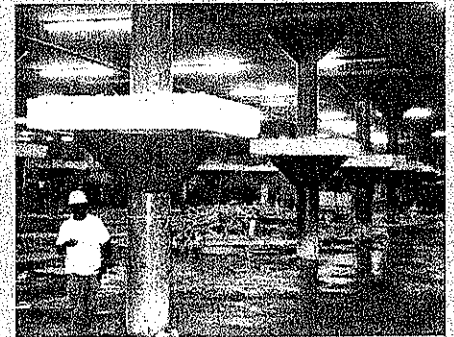
MCCORMICK PLACE PARKING TO REPAIR A SEVERELY DAMAGED PARKING STRUCTURE AT CHICAGO'S CONVENTION CENTER, WJE DESIGNED REPAIRS TO THE CONCRETE COLUMNS, REMOVAL AND REPLACEMENT OF THE CONCRETE SLAB, AND SYSTEM POST-TENSIONING.
