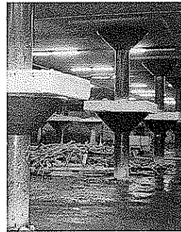
MCCORMICK PLACE PARKING TO REPAIR A SEVERELY DAMAGED PARKING STRUCTURE AT CHICAGO'S CONVENTION CENTER, WJE DESIGNED REPAIRS TO THE CONCRETE COLUMNS, REMOVAL AND REPLACEMENT OF THE CONCRETE SLAB, AND SYSTEM POST-TENSIONING.
