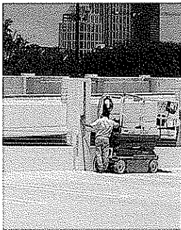
PARKING GARAGE REPAIR WJE WORKED AROUND THE CLOCK TO INVESTIGATE AND RECOMMEND REPAIRS FOR EXTENSIVE CRACKING OBSERVED AT AN ATLANTA PARKING GARAGE JUST AS IT WAS ABOUT TO OPEN.
