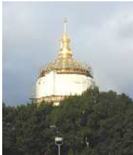
The white covering that has allowed work to continue through various weather conditions began coming down in early September.
